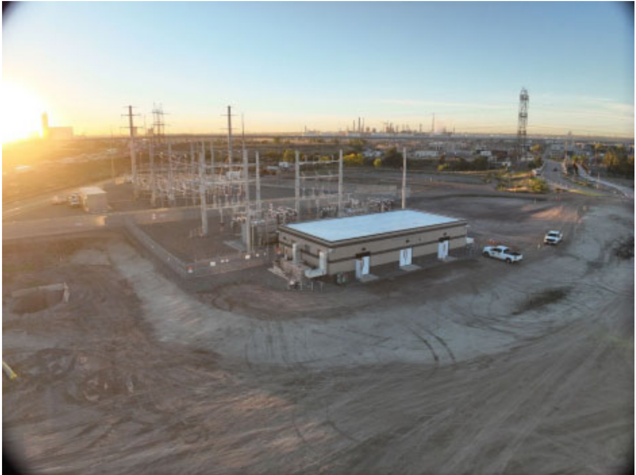
The new electrical transmission service substation at Robert W. Hite Treatment Facility.
