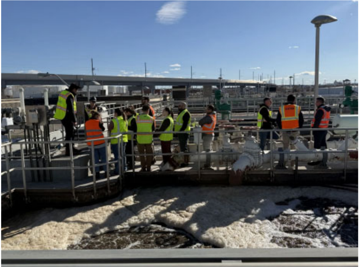
Tour group at the aeration basins at Robert W. Hite Treatment Facility
